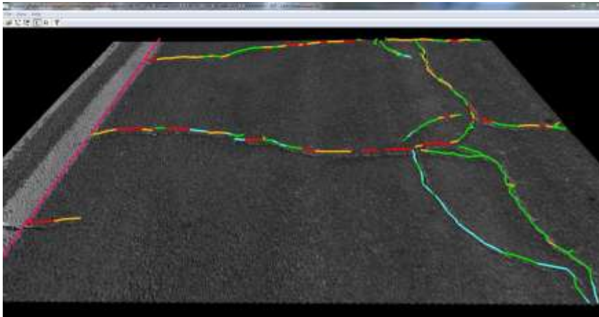
Figure 6. Example crack detection results (severity = color code).
