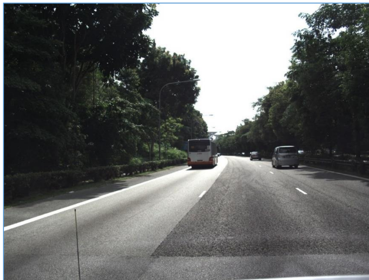
Figure 1: Ravelling Expressway Singapore
