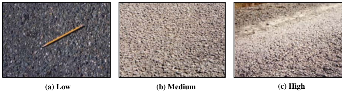
FIGURE 5 Raveling classification in WSDOT (WSDOT 1999).
