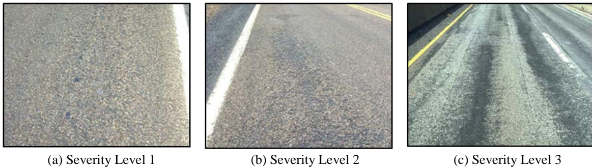
FIGURE 2 Raveling classification in GDOT (GDOT 2007).
