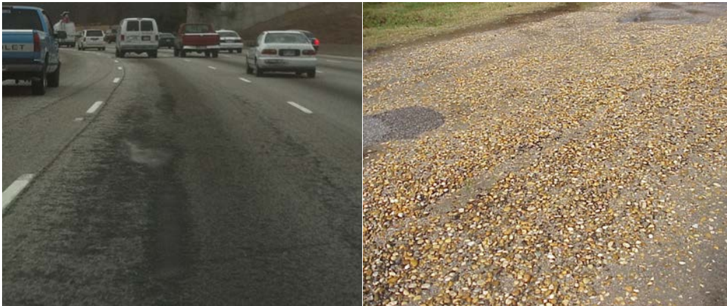
FIGURE 1 Raveling on interstate highway and non-interstate road.
